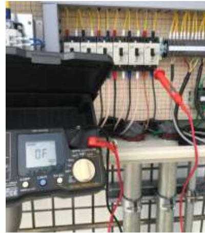
■ Insulation test – Pass Successfully!
