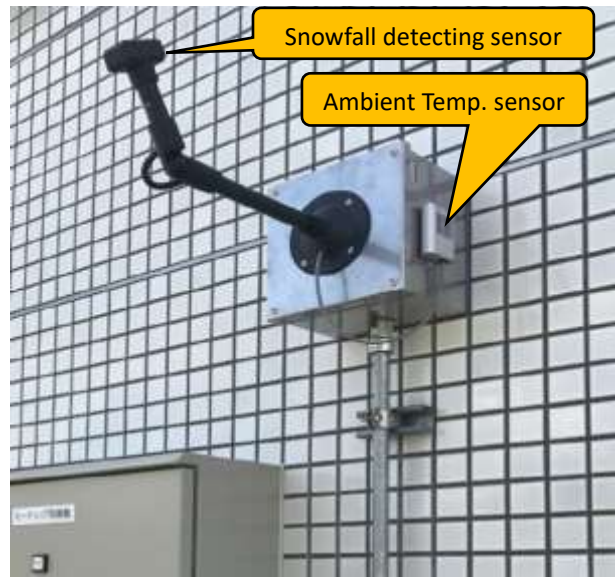
■ Control System's sensors
